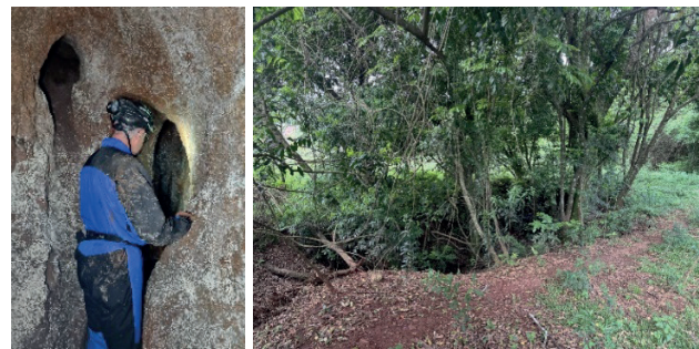
Figure 5: Conduit inspection; sinkholes.
